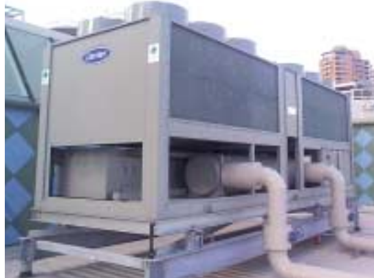
Air cooled chiller
